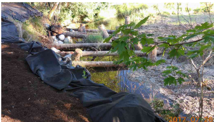
McLane Cr Accumulation Structure
